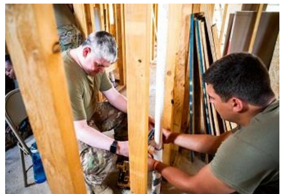
In 2023, The Air National Guard works together with Walking Shield, on a current housing rehabilitation and construction mission, to benefit the Blackfeet Tribe.
